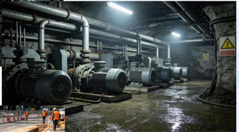
Mine pumping stations
